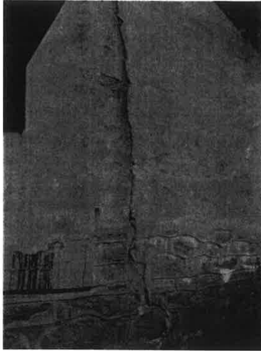
Photo 11 – Northeast Corner, Large vertical crack in the wingwall
